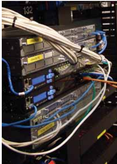
Uplogix creates an appliance which can monitor and diagnose problems with all of the amplifiers and modems typically involved in a VSAT communication system (pictured)
